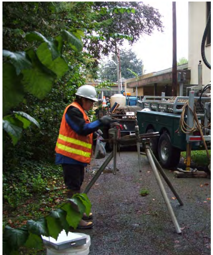
Susan Beckham of Associated Earth Sciences, Inc. evaluates core samples for soil bearing capacity at the Carnegie building this week
