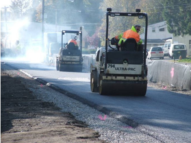
Paving machine placing steaming asphalt, followed by two roller-compactors on new section of Centennial Trail
